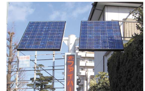
Solar power generation system
