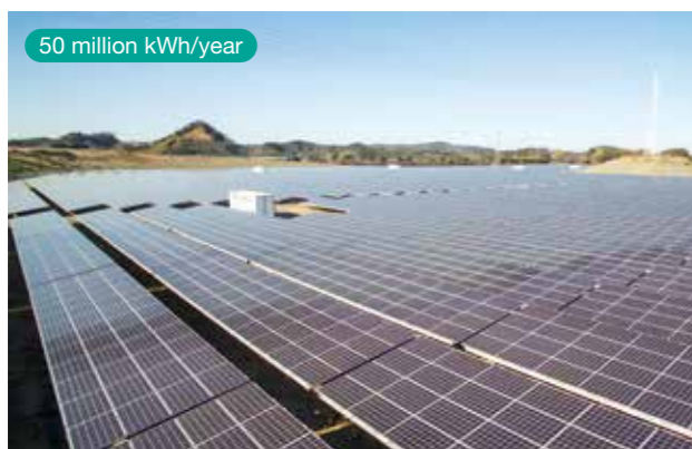
Green Power Futtsu Solar Power Plant (Futtsu, Chiba Prefecture)
