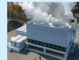
Geothermal power plant in Kumamoto Prefecture
