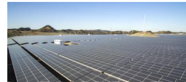
Green Power Futsu Solar Power Plant (Futsu, Chiba Prefecture) – 50m kWh/year
