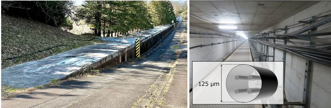
Fig. 4 Fiber installation environment within NTT Laboratories, underground facilities, and cross-section of multi-core fiber
